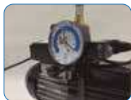
Connection with vacuum pump
